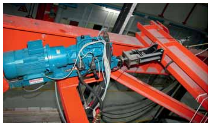
Actively controlled actuators
