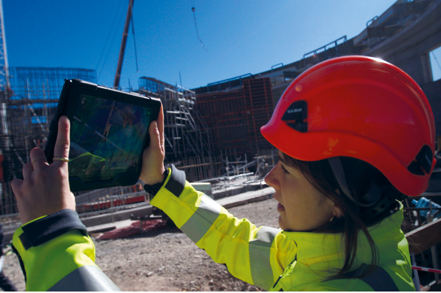
A worker on the ELT construction site holds a tablet computer, used for an augmented reality system that assists with the installation of components for the ELT's dome and main structure.
