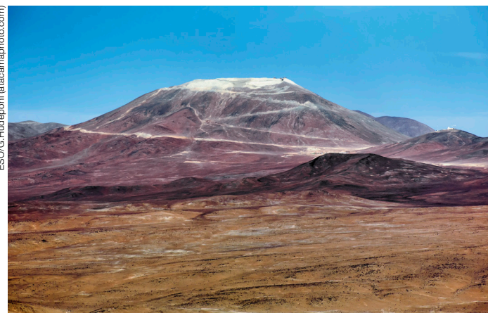
Rapid progress in flattening the peak of Cerro Armazones had been achieved by December 2014.
