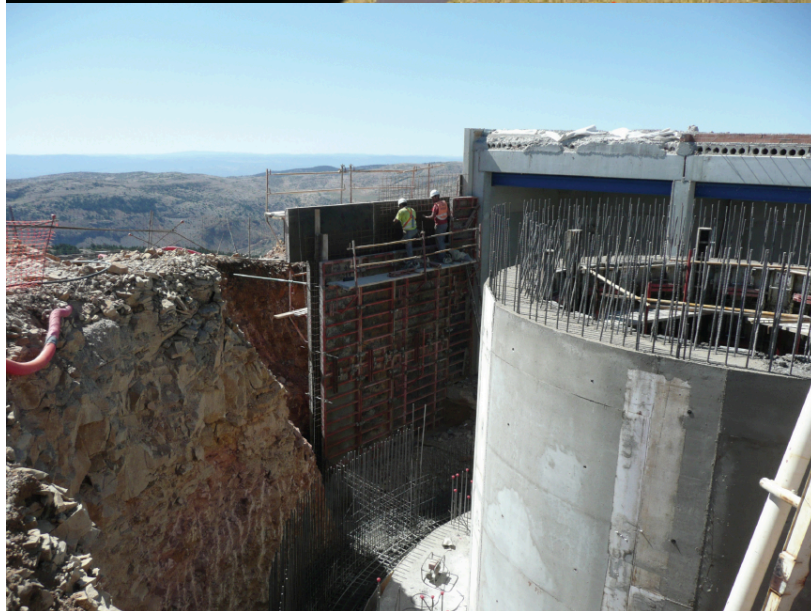
Control Room & Laboratories
