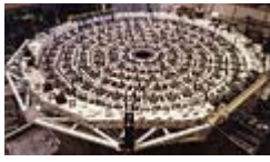
Figure 4.3 [JPG: 312k]. The M1 active supports, during the installation into the M1 Cell.
