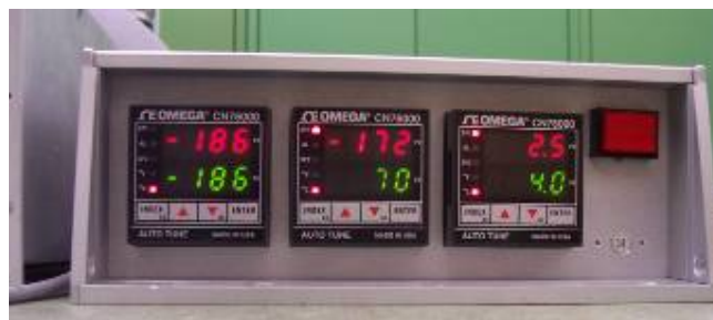
Figure 8 - The OMEGA controllers box
