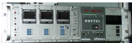
Figure 83 Vacuum pump controller
