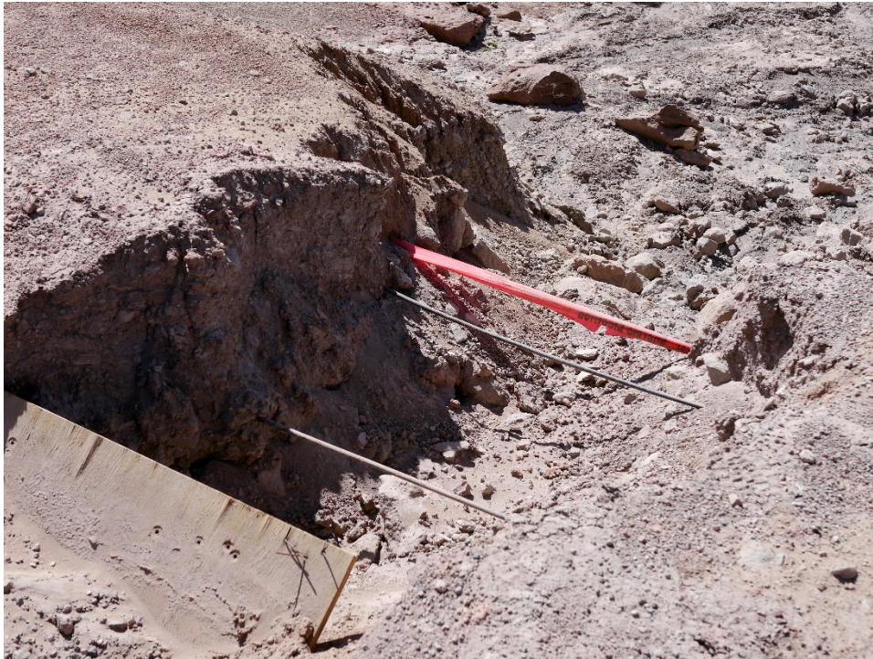
Figure 15 Exposure of the fiber cable between one antenna pad and the AOS
